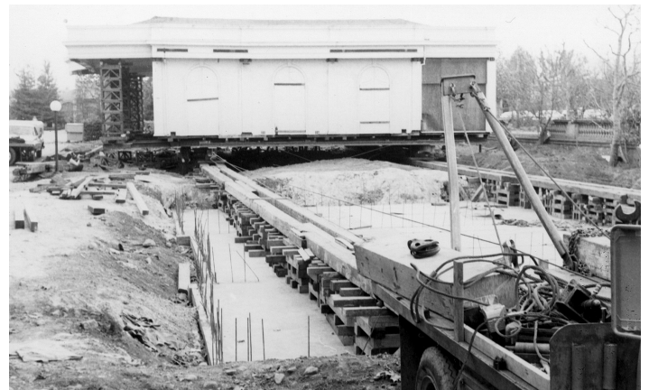
In 1974 the Trianon was moved from a temporary position on cribbing in a parking lot to its present site after five years of fundraising for its rehabilitation.
